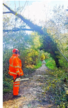
Removal of a wind damaged tree at the Res & below damaged tree on the far side of the Res.
